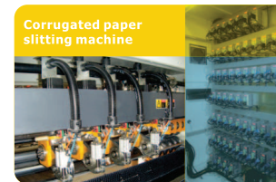
Kinco provide total CANopen solution in Corrugated paper slitting machine
